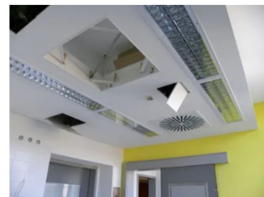
CLEAN ROOM HEPA FILTER REMOVED
